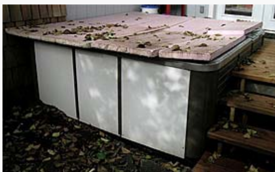
Poorly fitted or improper spa cover
